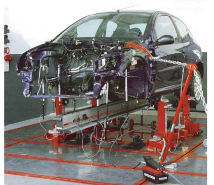
Used in conjunction with a frame correction machine. The movement of the frame when pulling is visible.
